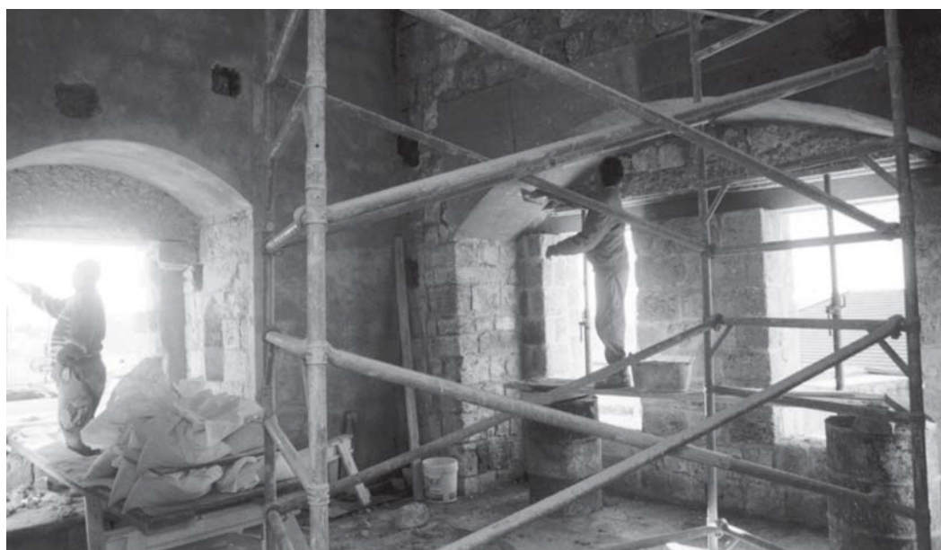
The restoration work in the room once occupied by Bahá'u'lláh. Many measures were taken to ensure the sacred and historic character of the citadel was respected.
